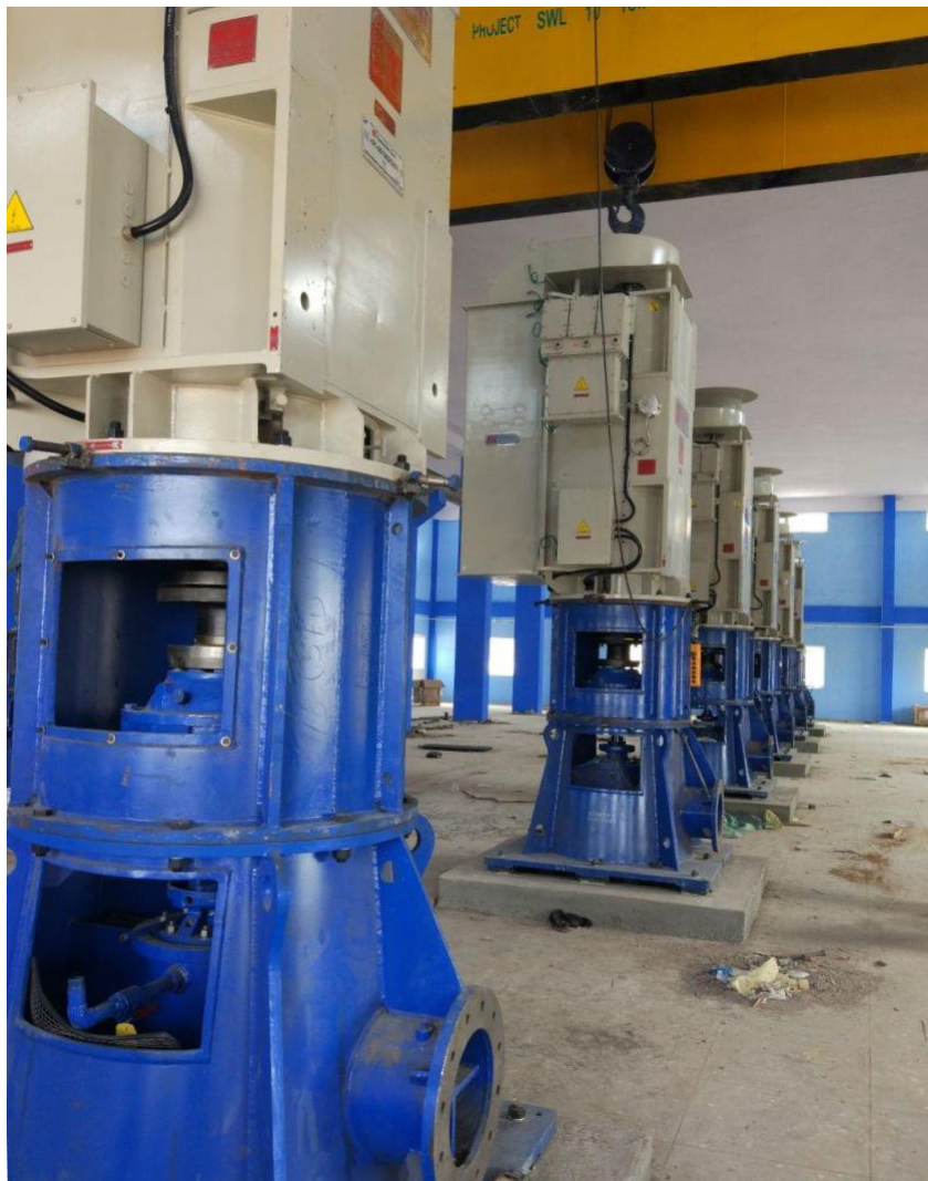
Pumpsets @ Mallannagutta WTP
