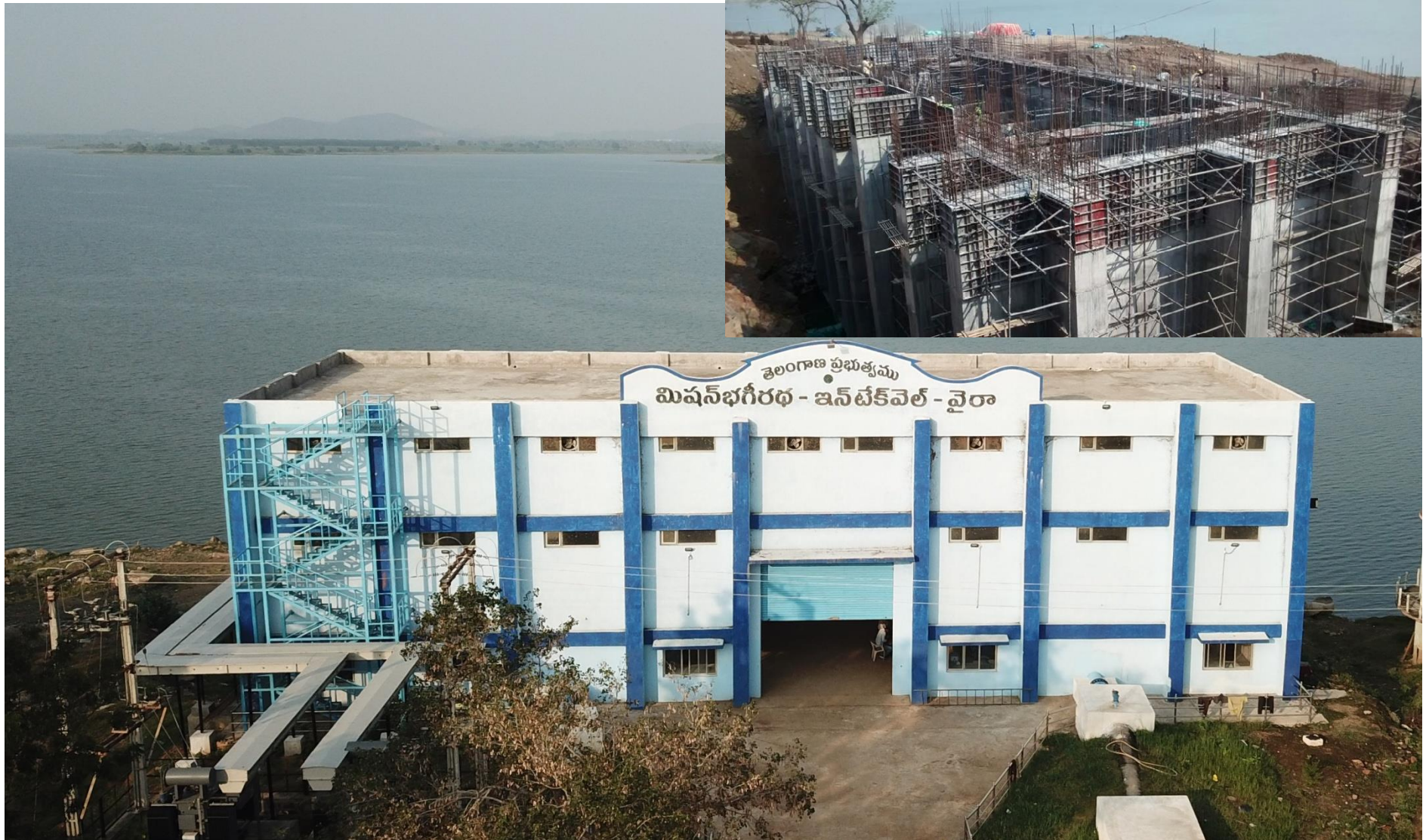
Intake well @ Wyra Reservoir
